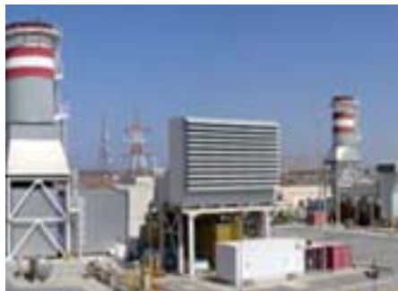
Barka Power Plant - Oman
